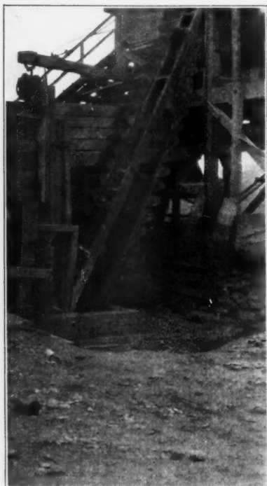
Detail of Elevator from Crusher to Scalping Screen.
